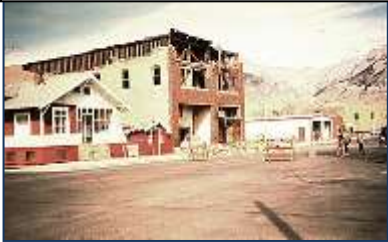
Unreinforced masonry buildings are susceptible to shaking and create debris.
