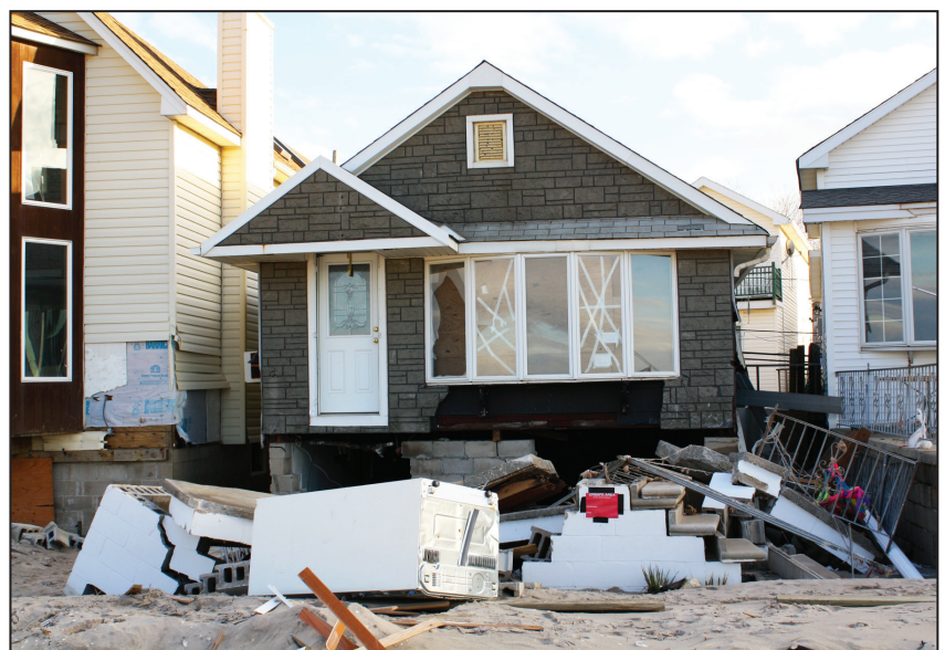
Figure 5: Elevating tightly spaced homes, such as these in Breezy Point, NY, presents construction challenges.
