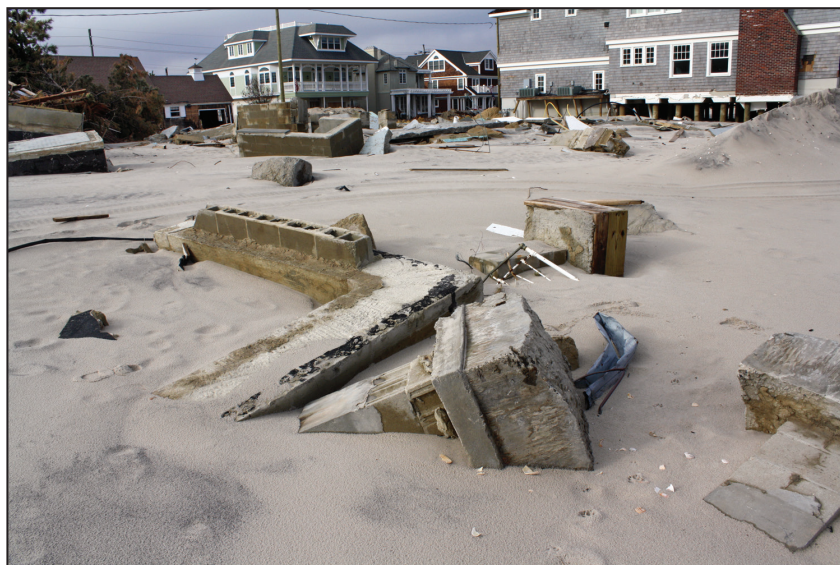
Figure 6: Discrete pier footings undermined by erosion and scour in Mantoloking, NJ.
