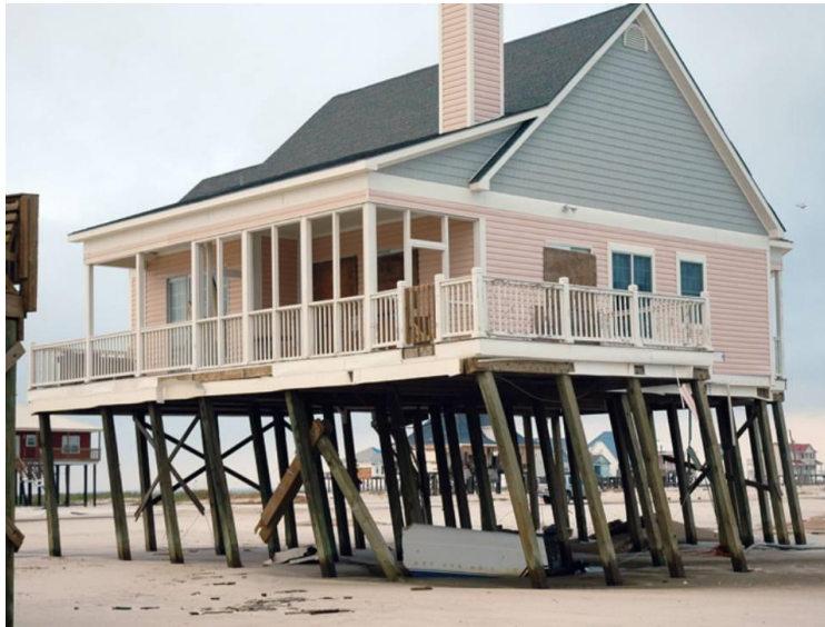
Figure 5-3: House on verge of collapse due to shallow embedment of timber pile foundation
