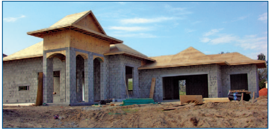
CMU was used for the exterior walls at this house under construction (New Smyrna Beach, FL).
