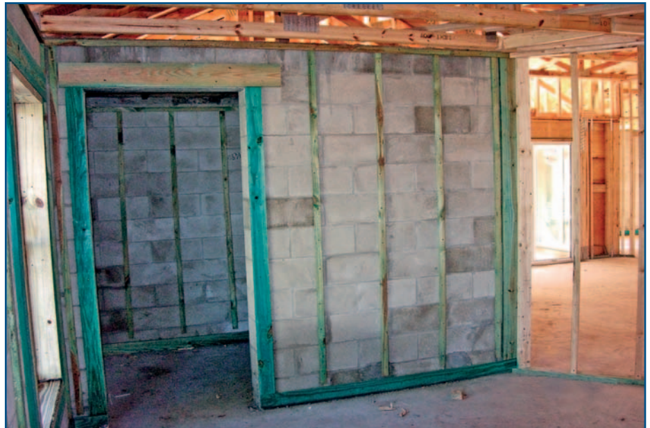
View of an in-residence safe room under construction. Steel reinforced and fully grouted CMU surround the safe room space (New Smyrna Beach, FL).
