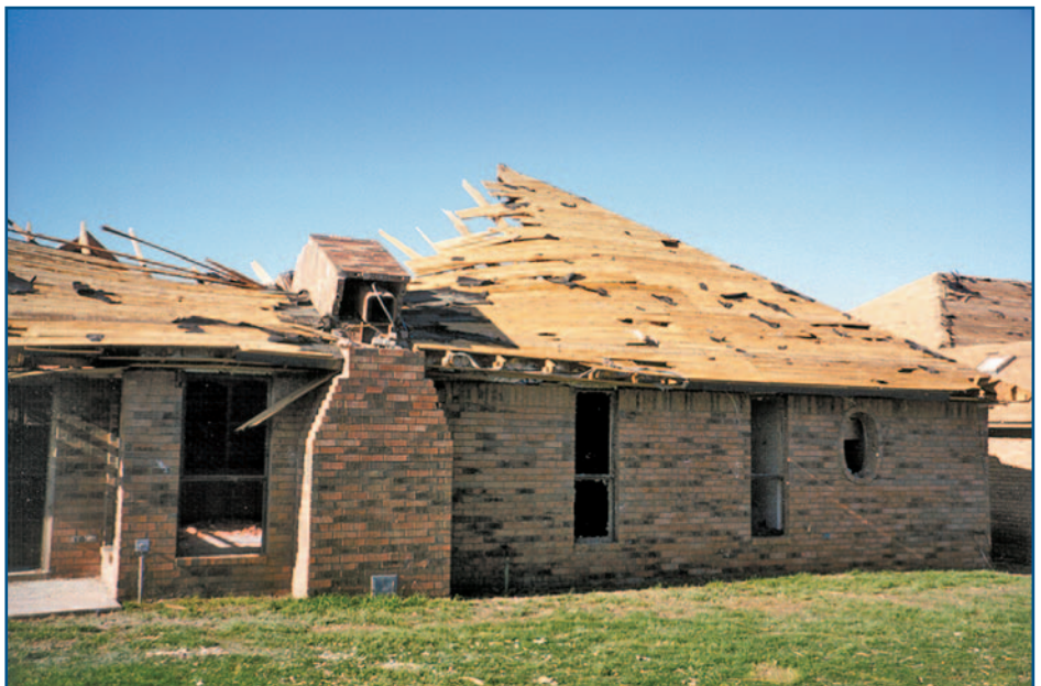
Avoid selecting a refuge area that is near a masonry chimney (Moore, OK).
