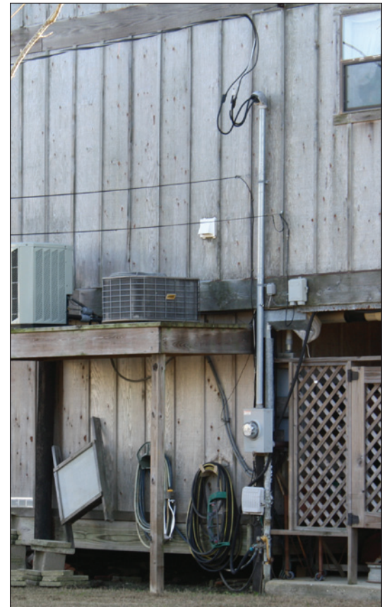
Figure 1. Electrical components installed below the lowest floor system are subject to increased flood damages and lengthy outage durations (St. Tammany Parish, LA)
