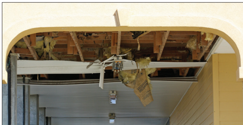
Figure 1. Loss of the covering from the underside of an elevated building due to high winds (Plaquemines Parish, LA, Hurricane Isaac)
