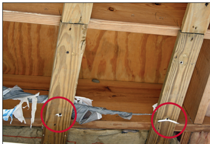
Figure 3. Covering under an elevated building was lost when the vinyl soffit paneling tore around fastener heads during high winds (Plaquemines Parish, LA, Hurricane Isaac)
