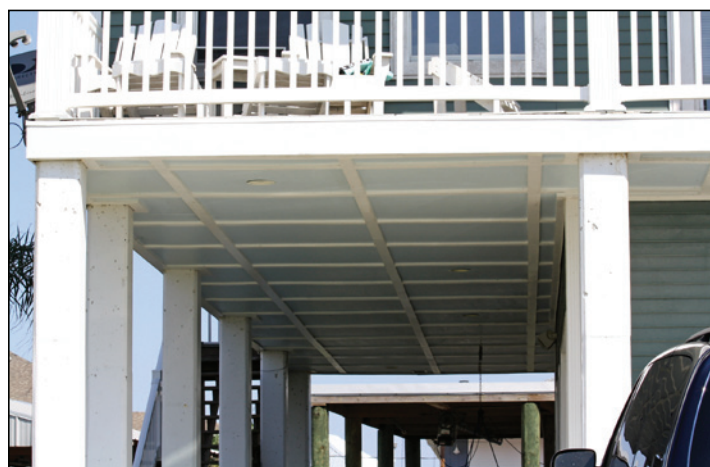
Figure 4. Wood sheathing under a house near the one shown in Figure 3 did not fail; this is not a fire-resistant-rated assembly (Plaquemines Parish, LA, Hurricane Isaac)
