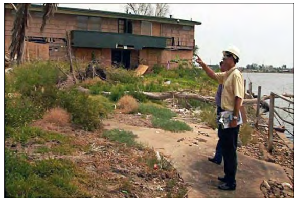
Figure 2-3: Screening the exterior of a damaged structure
