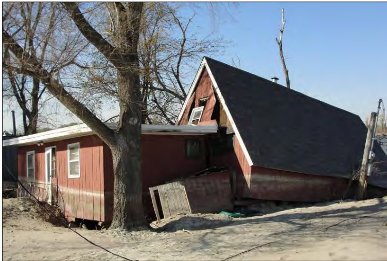
Figure 4-1: Two views of the same structure showing a high water mark, structure displacement, and some of the damage
